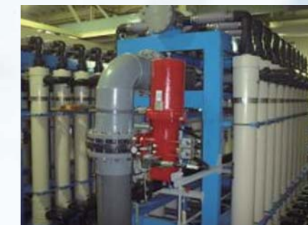
Seawater Desalination (for RO pretreatment) Capacity: 2,700m 3 /d Location: Ehime, Japan Operation start: Sept. 2003
