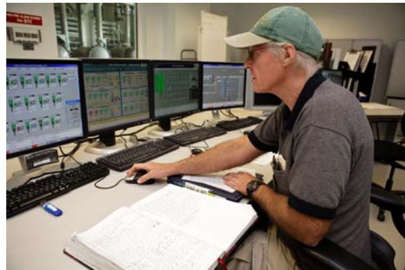
WWTP Control Room
