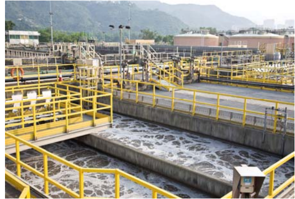
WWTP Aeration Tanks
