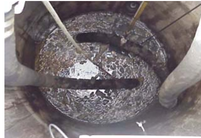
Crown Point, IN Lift Station Prior to IPT Treatment
