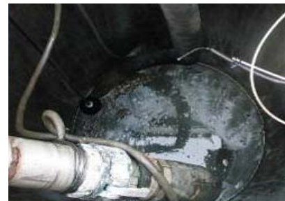
Crown Point, IN Lift Station With IPT Treatment
