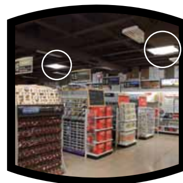
Retail store with SunWave SMRT lighting
