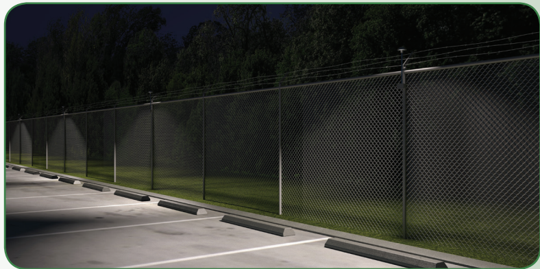
Typical perimeter lighting application.
