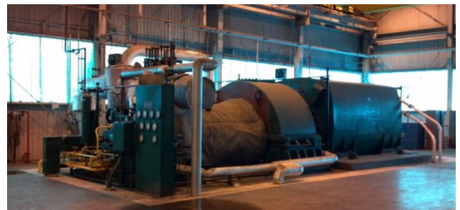
Former Boralex / Sherman 24 MW Power Plant Turbine in Stacyville.
