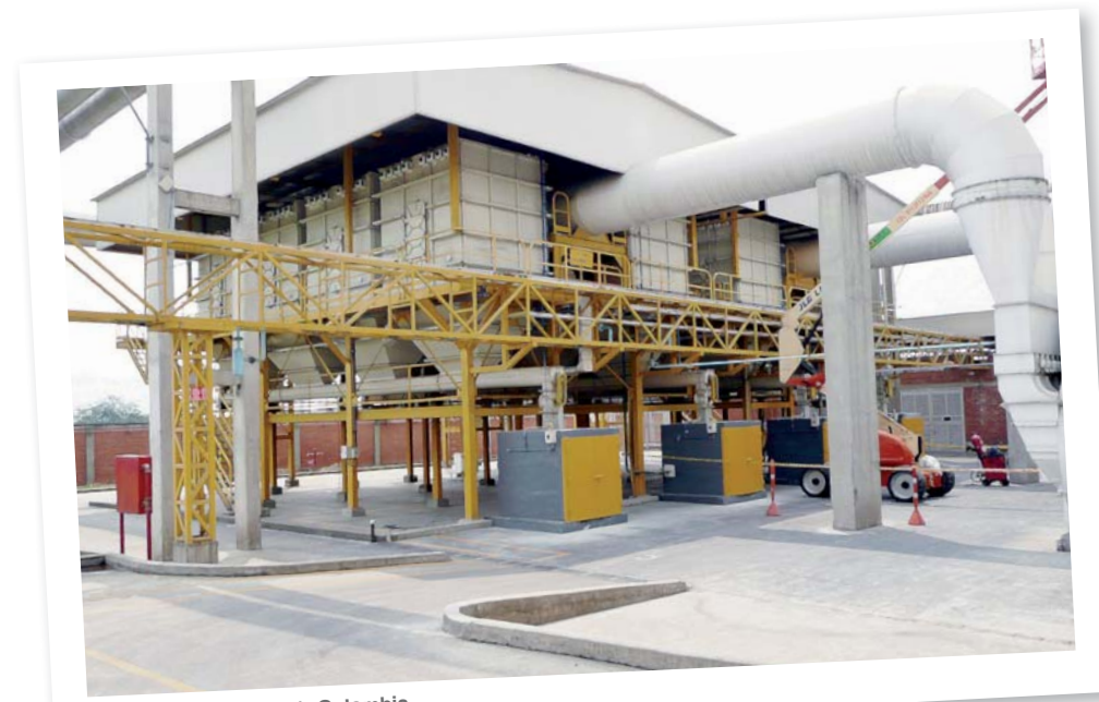
Filter Plant (Baghouse), Colombia
