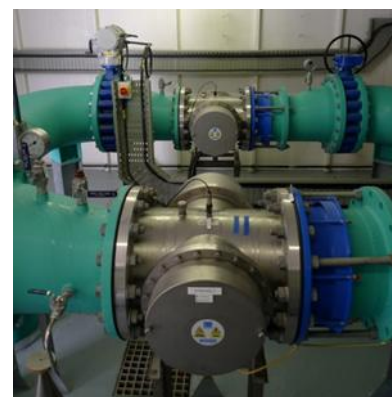
ETS UV model SX installed duty/standby
