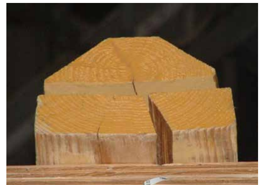
Wood chocks will crack, split, splinter, warp, and rot over time
