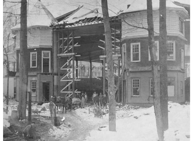
c. 1907 photo during installation of the Massey Organ, shows original towers (now hidden)
