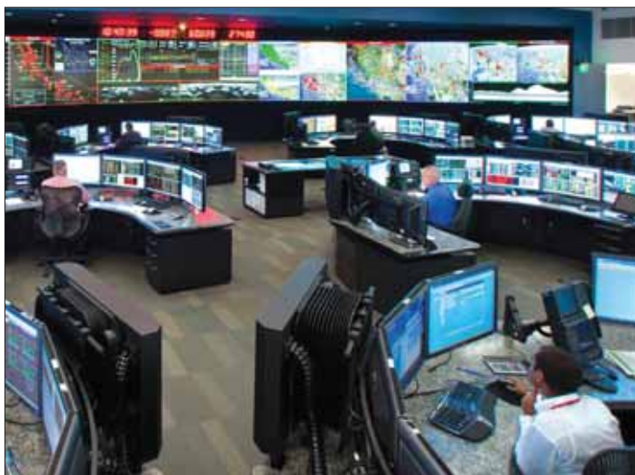
The control room at CAISO. COURTESY CAISO.
