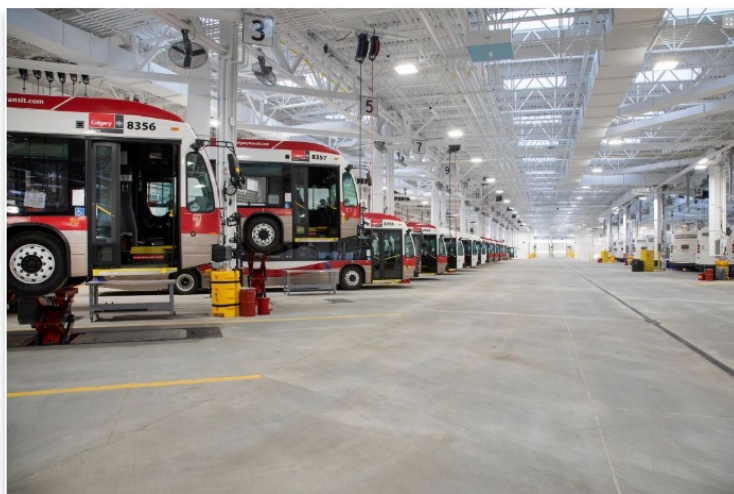
Stoney Transit Facility service bays are equipped with Stertil-Koni scissor-style ECOLIFTS, supplied by Westvac Industrial. Photo courtesy of the City of Calgary.
